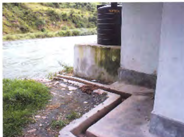
Photo 11.2 Drainage from public toilet
